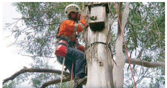
A worker is installing a nest box to provide the habitat for local wildlife.
