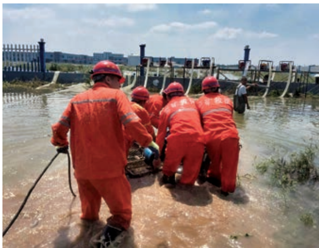
Rescue work at Shouguang
