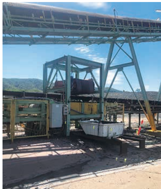
Raw Coal Washing System at the Washery of Yancoal Australia Limited.
