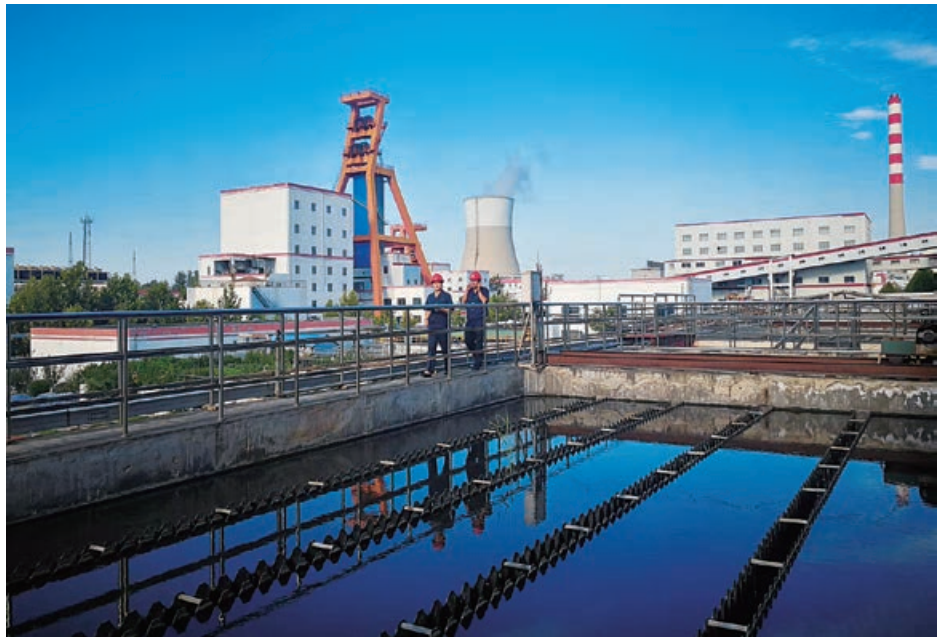
High-standard sewage treatment tank
